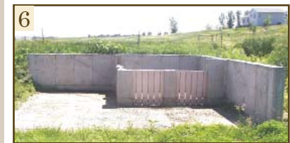
Solid separator separates solids from run-off water and allows dirty water to run into the evaporation pond.
